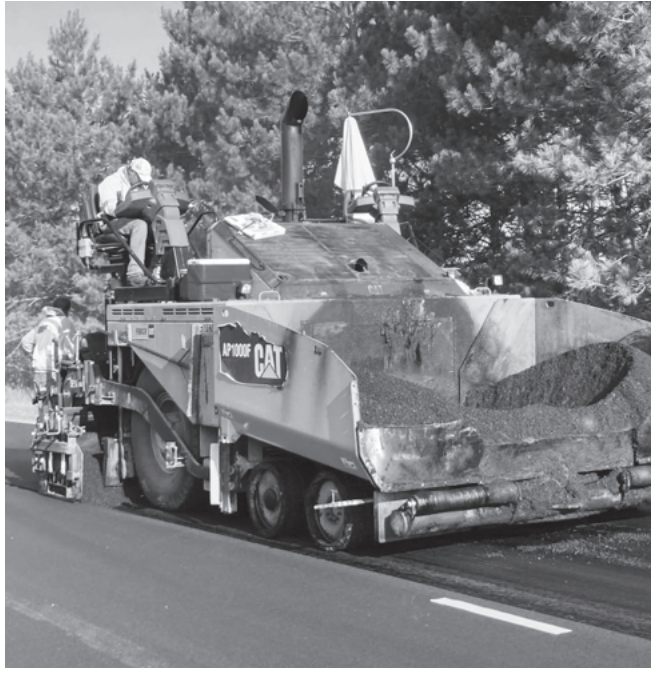
Rubber-modified asphalt that uses recycled tires is being used to pave some highways in Michigan.
